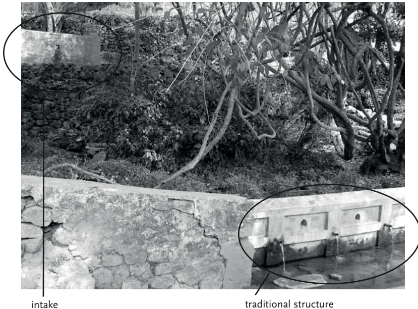
Figure 3.2 Positioning of intake in relation to traditional structure. Photograph by Monique Mikhail.
